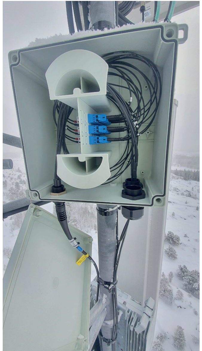
Figure 1 – FTTA distribution box mounted on communication tower in winter conditions
